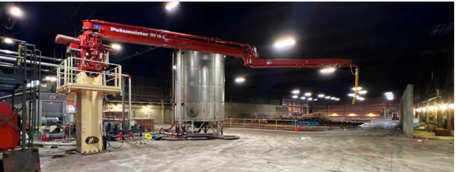
Loading arm and storage tank in background
