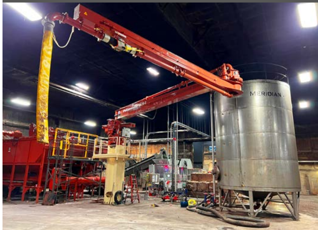
After installing RV 16 and EQV on loading arm with paste and slurry hoppers in the background, liquid storage tank on the right
